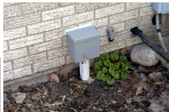
Buried PVC for coax entry into house.
