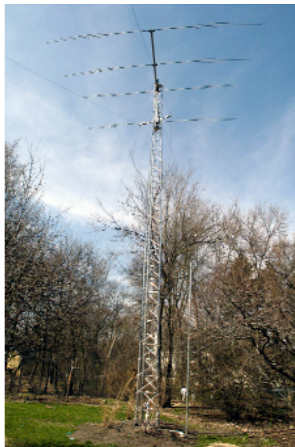
Tower nicely blends in with surrounding vegetation.
